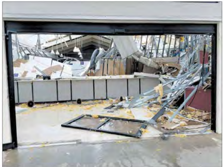
Sunlight lights the inside of the Frenchtown Post Office on Thursday afternoon after winds from Hurricane Irma ripped the roof off the building.
