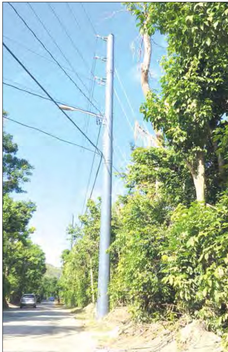
A composite pole installed in the Adrian area of St. John.
