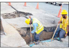
V.I. Water and Power Authority employees Miguel Wilbering, left, and Djour Shoy repair a broken water line Wednesday on St. Thomas.
